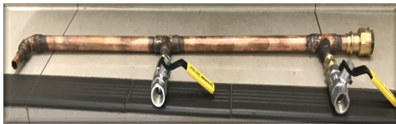
Figure 5: multiple appliance manifold
