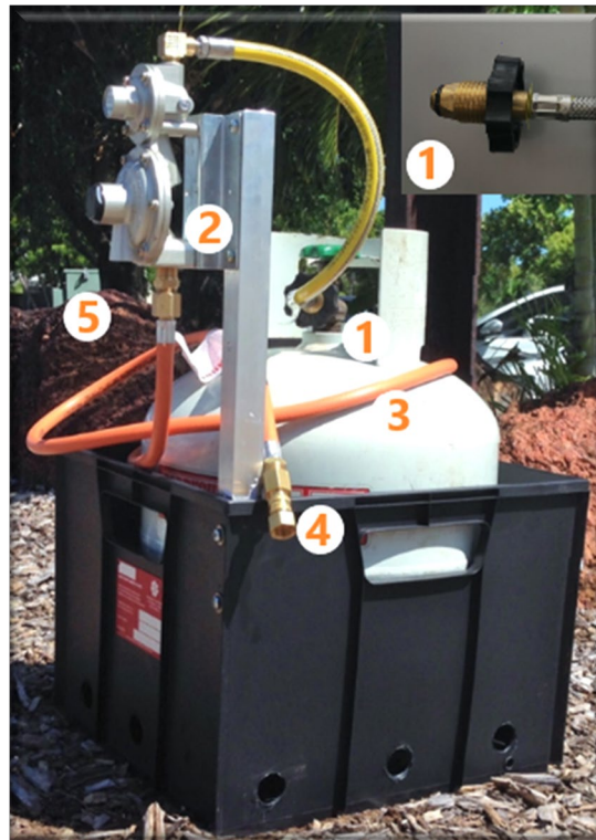
Figure 2: One LP Gas Cylinder for one appliance with low consumption rate
