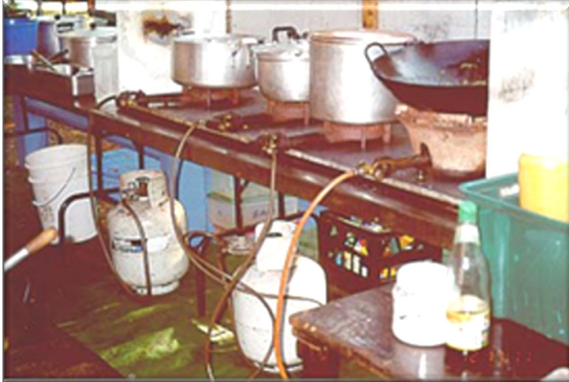
Figure 7: Examples of unsuitable and possibly very dangerous appliance installations.
