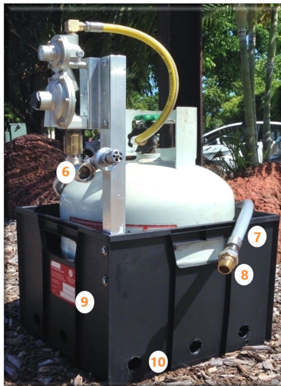
Figure 3: one LP gas cylinder for multiple appliances via manifold
